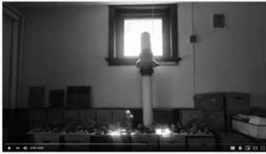
radon mitigation apparatus
